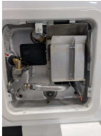
Water Heater Open
