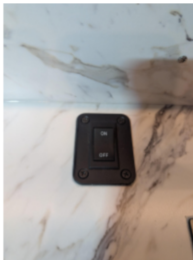
Water Pump Switch
