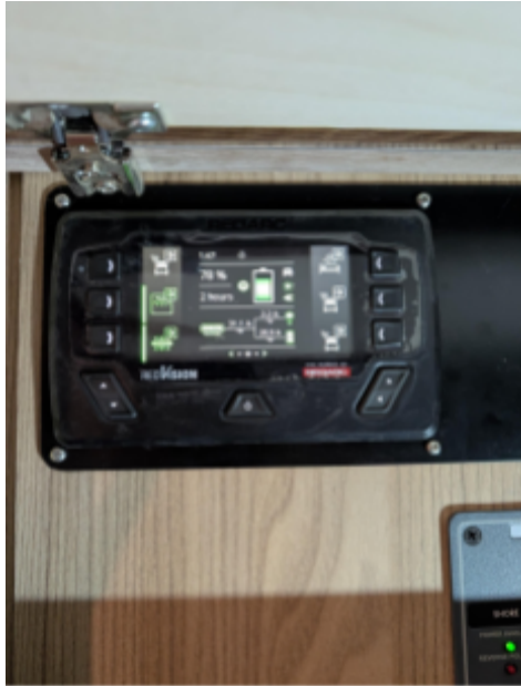
RedVision Battery Monitor
