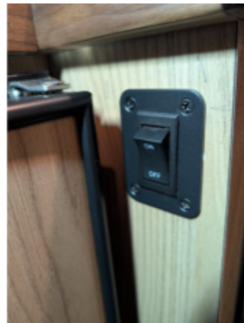
Sump Pump Switch
