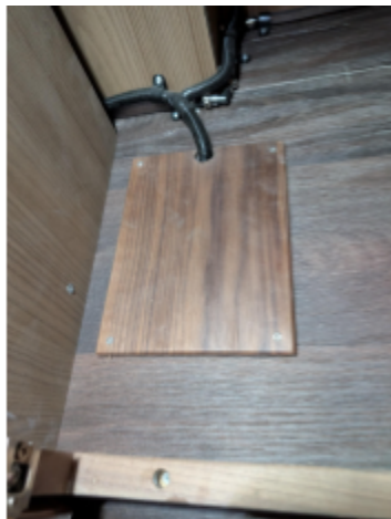
Sump Pump Location (under false floor)
